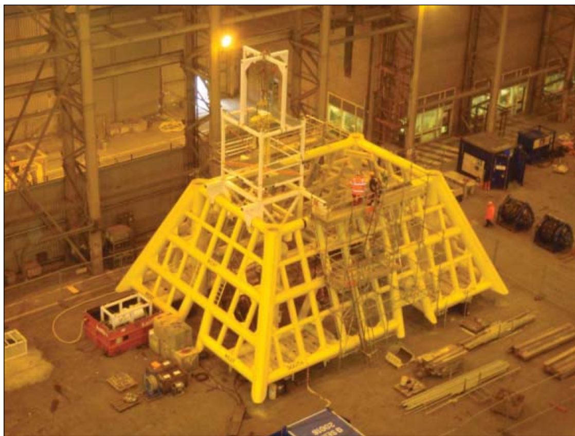
Preparation for the offshore hot tap included system integration tests at the BiFab yard, Methil, UK. The hot-tap machine—with the hot-tap valve attached—was lowered from the hot-tap installation frame (in white) into the subsea protection frame. Once situated in the protection frame, engineers supervised connection of the hot-tap machine and valve to the hot-tap nipple for pressure testing before performing the hot tap (Photo by T.D. Williamson; Fig. 1).
